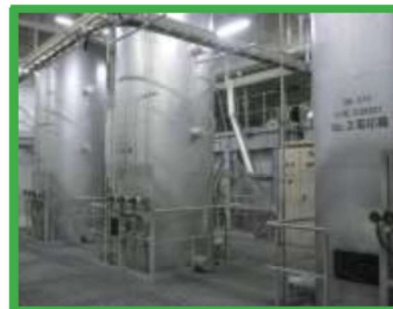
▲ PCB decomposition reactor
